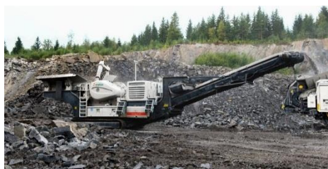
Figure 1. Concrete Recycling plant
