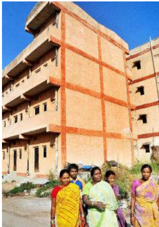
Figure 1: Multistoried row VAMBAY housing at Hyderabad.
